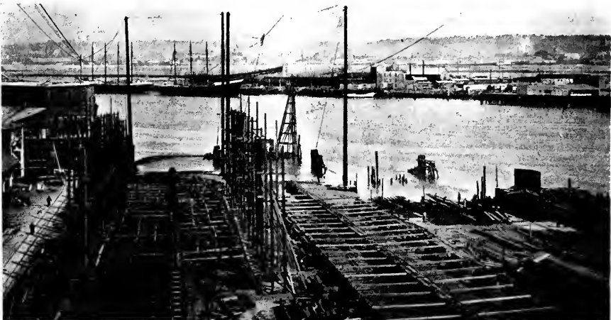
Laying out keel-blocks and building-ways, showing the overhead trolley handling system employed in handling material.
